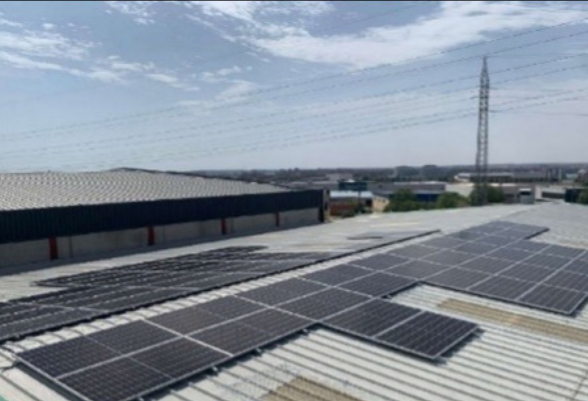
Solar panels at Intersurgical Spain
